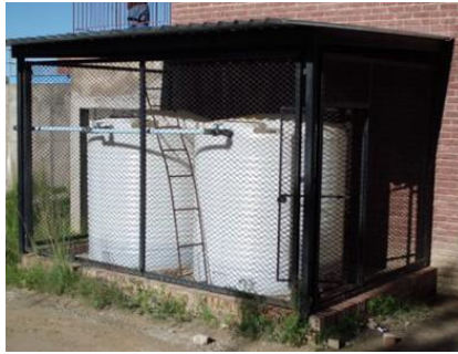
Main holding tanks for flocculent at the Hobhouse WTW
