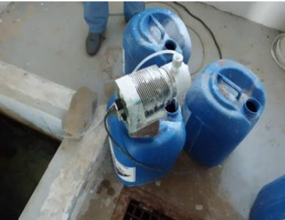
Chlorine dose pump balanced on sodium hypochlorite drums
